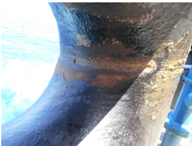
Figure 4.2.2/1: The part of the closed chock against which the rope passed during the mooring operation.
